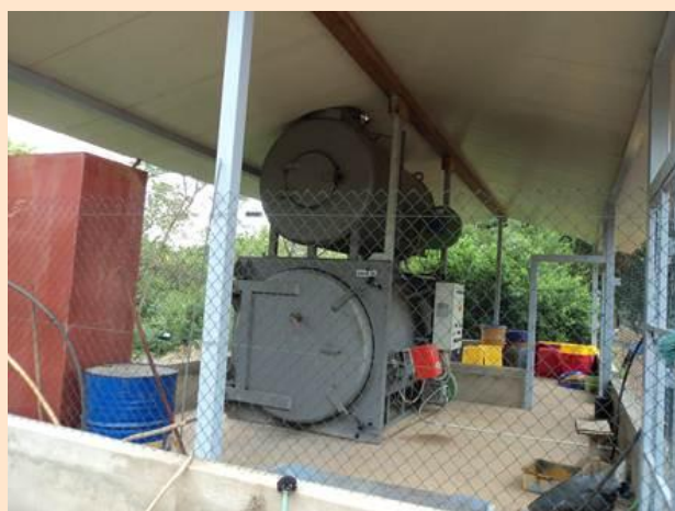
A double chamber incinerator of St. Jean de Dieu Hospital of Languieta
